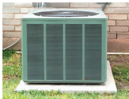
This air conditioner transfers heat energy from the cool indoors to the hot exterior.
