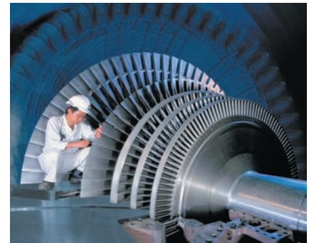
The steam turbine in a modern power plant is an enormous device. Expanding steam does work by spinning the turbine.
