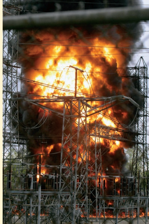
■ FIGURE 13.28 Fire that broke out in 2004 at the 340,000 V American Electric Power Substation near Mishawaka, Indiana. (© AP/Wide World Photos)
